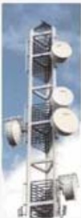
Aesthetic tripole structure
